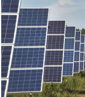
A row of solar energy panels. Photo Credit: Brookhaven National Laboratory/Flickr
